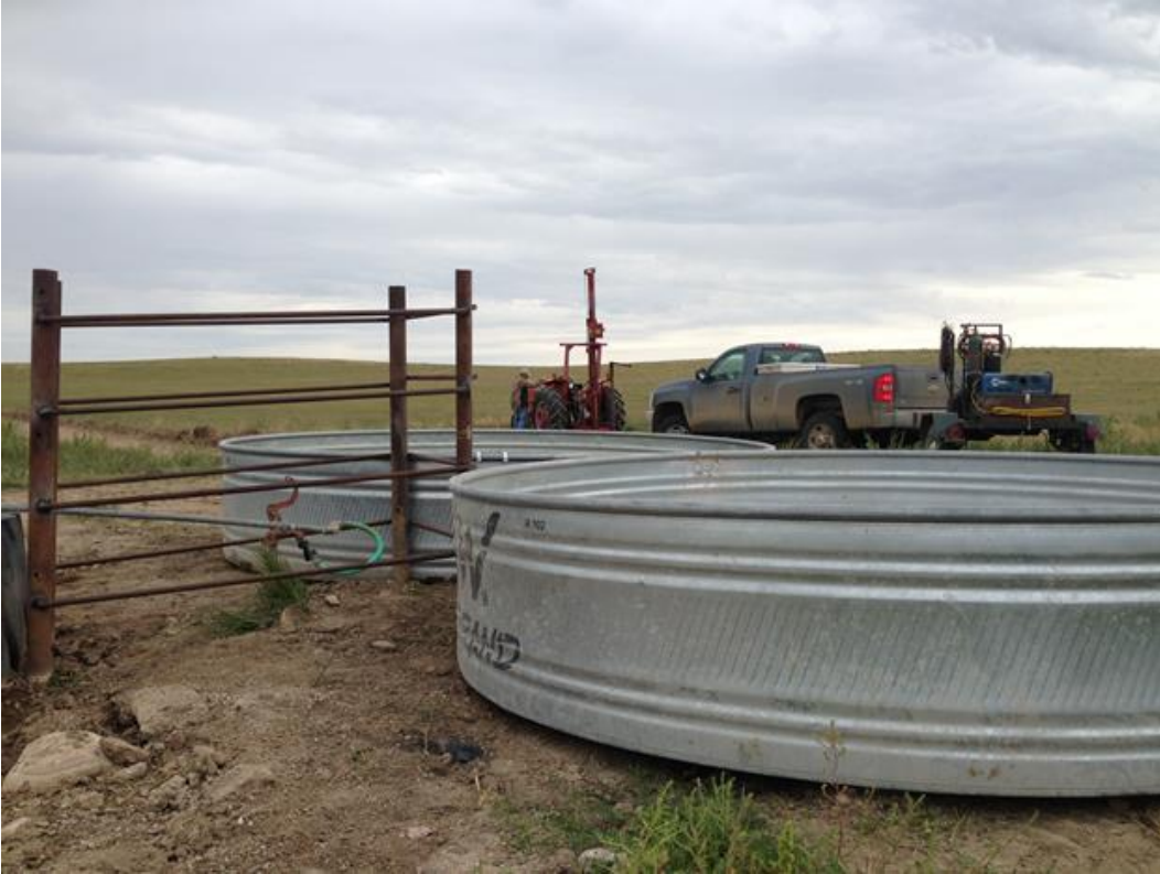
The CPER crew finishing repairs and installation of two new water tanks in the Crossroads pasture.
